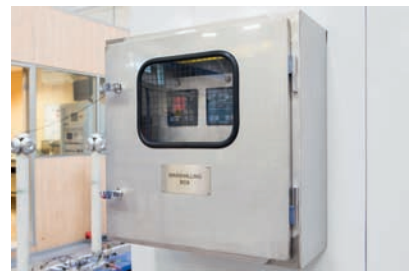
External Marshalling Box
