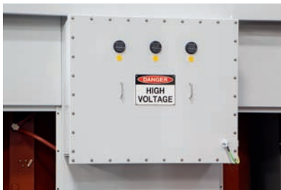
Cable Box with Infrared Windows
